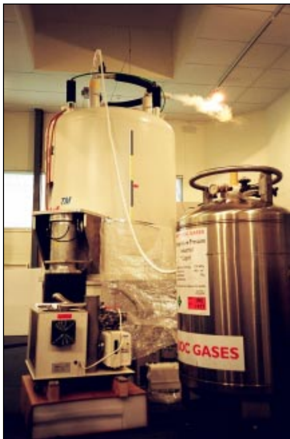
The installation commences with the introduction of liquid nitrogen to start the cooling down process
