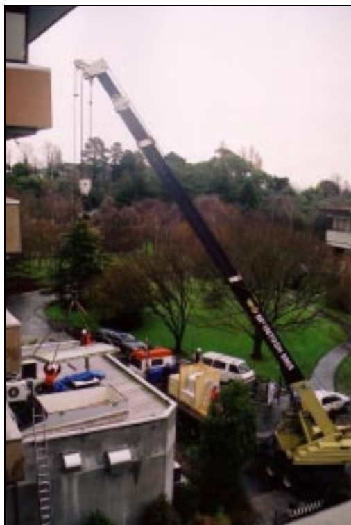
The roof does come off
