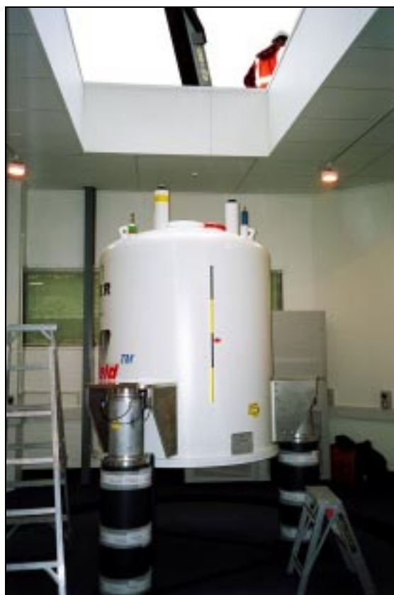
700 firmly bolted to the support mounts and the floor
